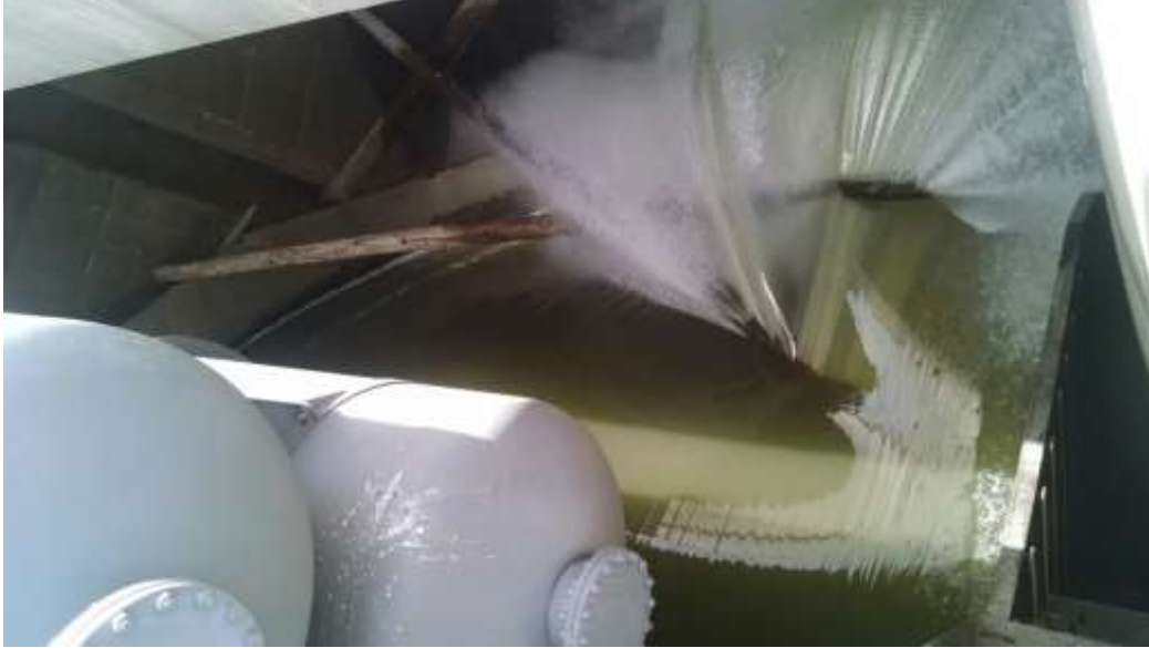
Photo 2. Logs across RSW prior to gate operation.
